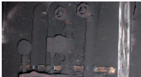
Fire damage before ...
