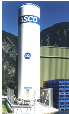
Vertical CO 2 storage tank
