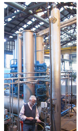
High Pressure Purifier
